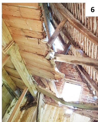
6 – Decaying roof of the Sacristy
